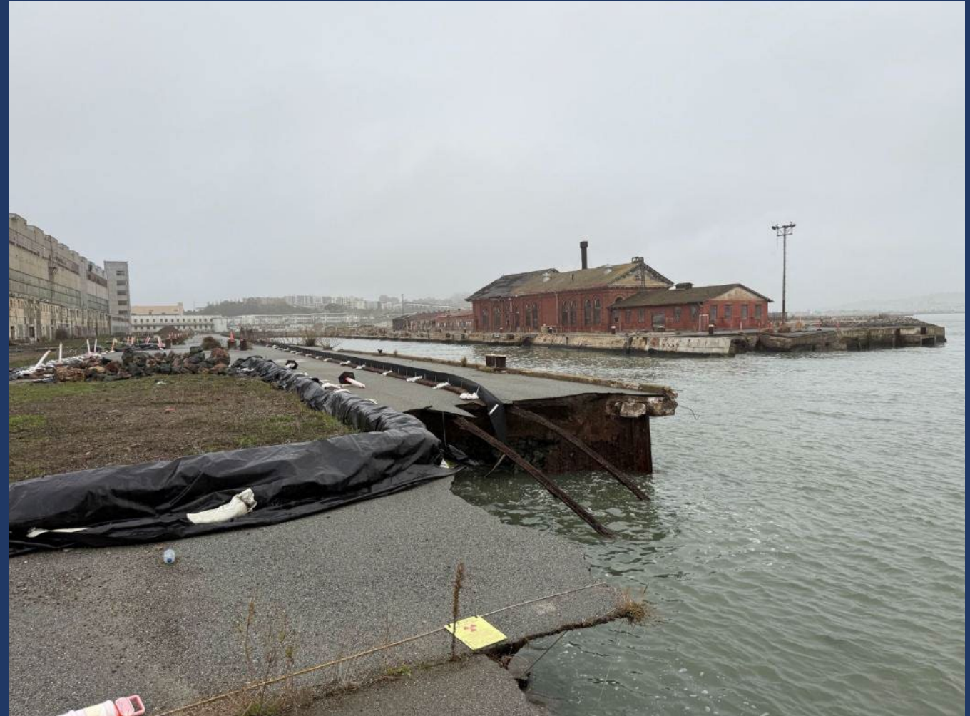
Close-up view of eroded dry dock, Parcel C
