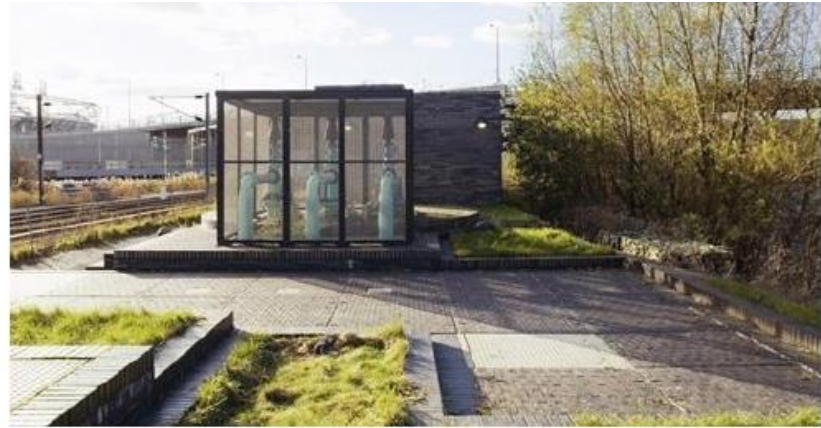
STRATFORD BOX PUMPING STATION, LYALL BILLS & YOUNG, STRATFORD LONDON, UNITED KINGDOM
