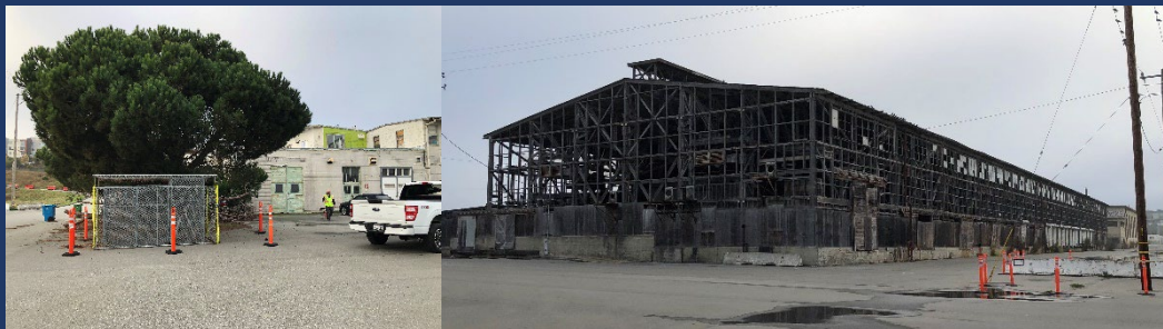
Air Monitoring Station at B116 and Building 123
